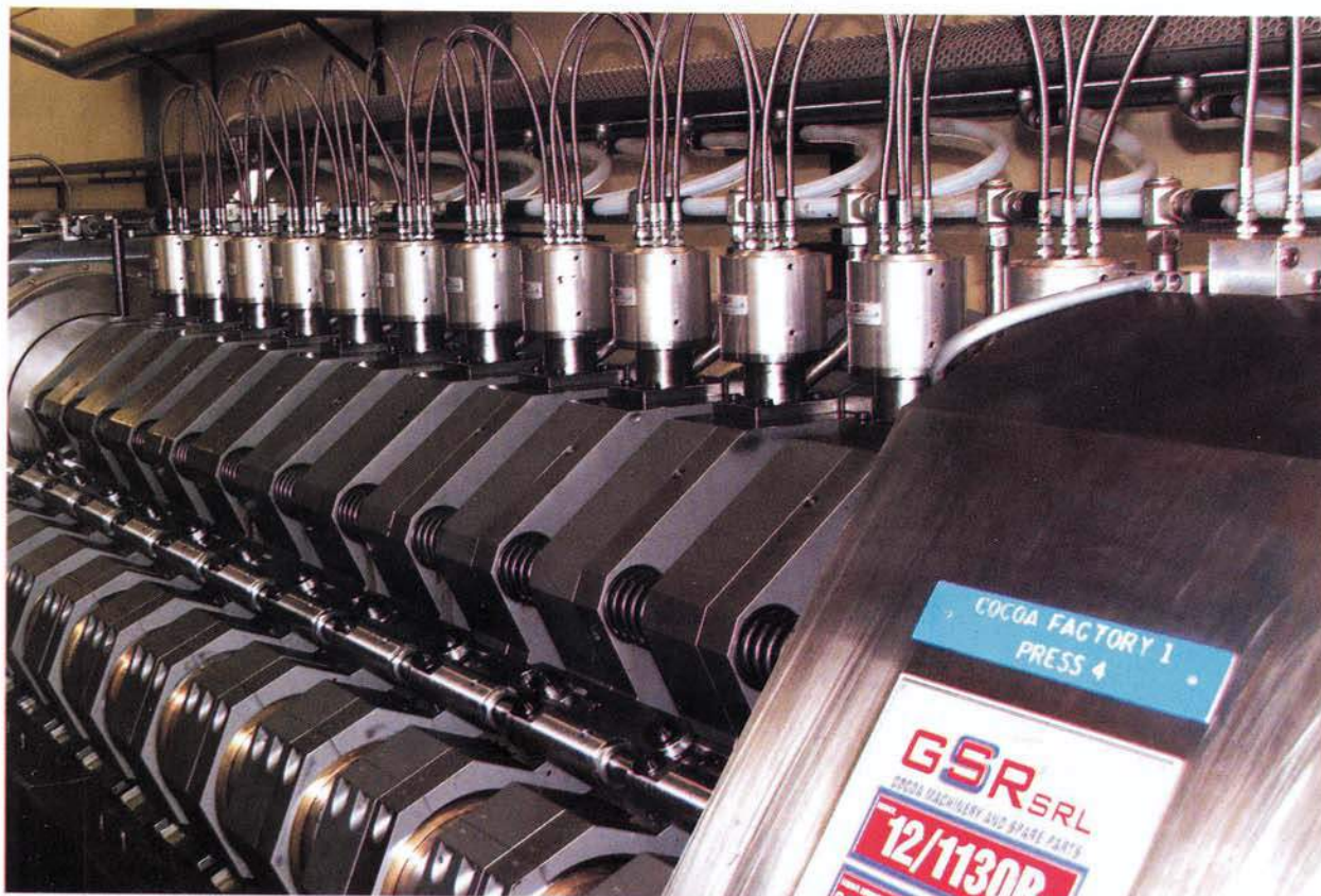
One of the new, state-of-the-art butter presses installed at the newly refurbished and upgraded Cocoa factory
