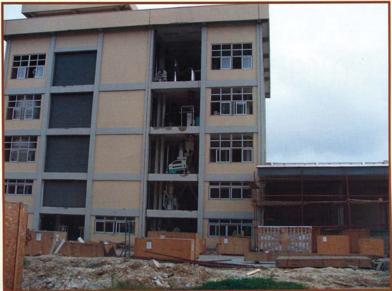
Front view of the new CPC Factory being constructed as part of the expansion programme.
