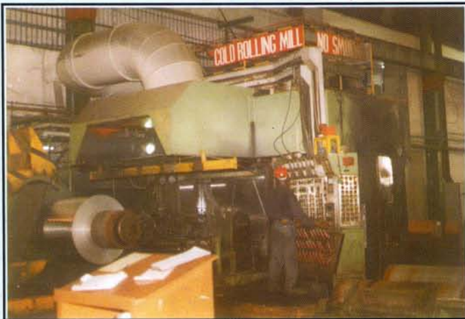
Cold Mill, a key Machine in the Plant
