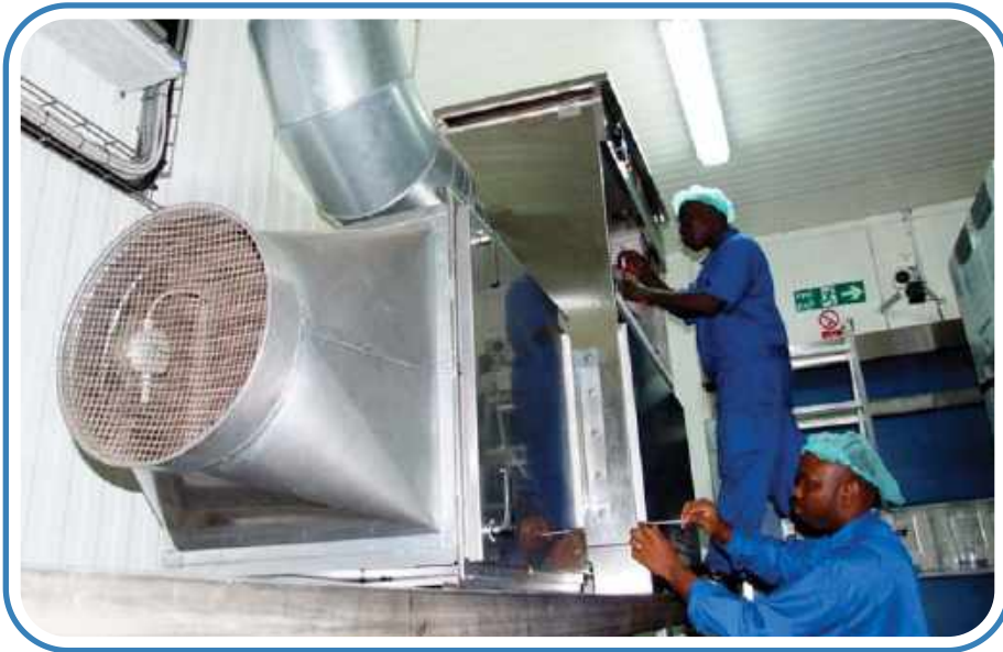
New dehumidifier equipment.
