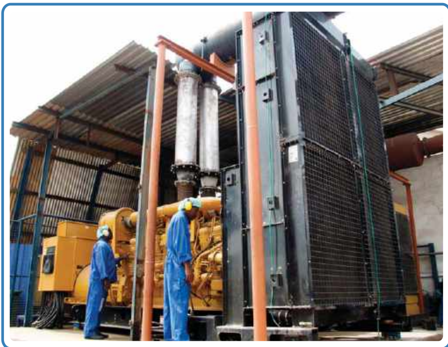
Newly installed 2MW Generator plant.
