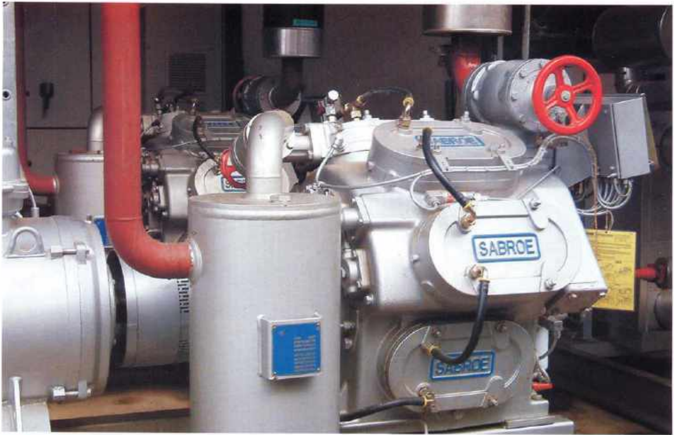
Water Chiller Compressor.
