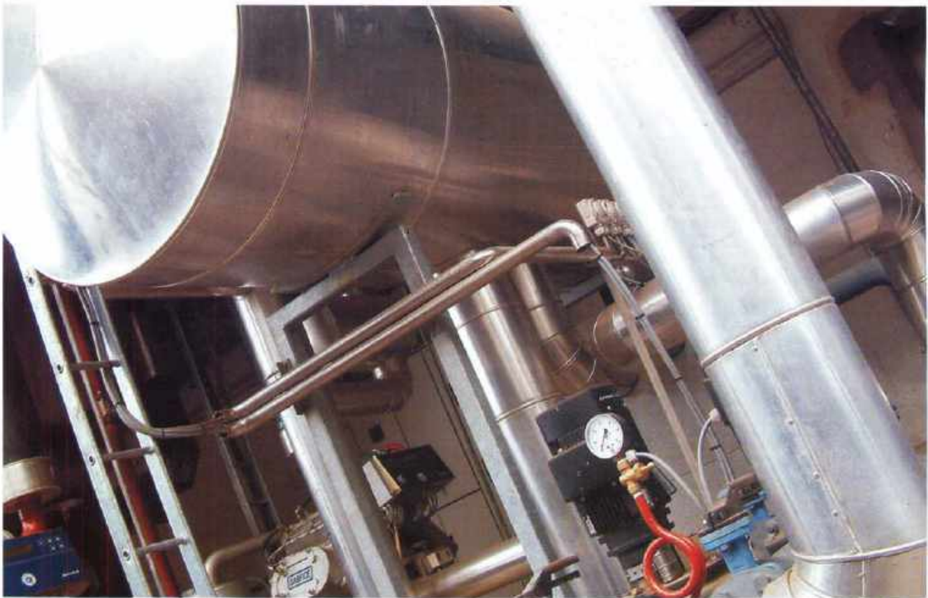
Water Chiller System.
